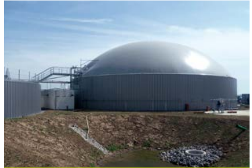
Biogas plant Schöntal-Bieringen
